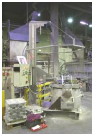
Heizstation elektrisch Electrical heating station
